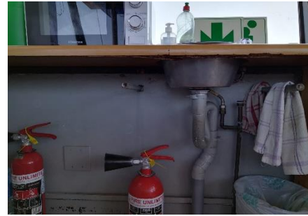
Figure 48. FAVG sink and tap plumbing
