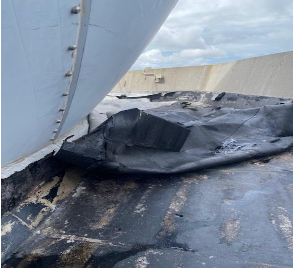
Figure 1: Example of an area that requires refurbishment.
