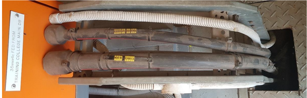
Figure 5: Generator power cables
