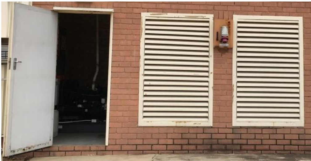
Figure 4: Entrance and mobile generator plug in port
