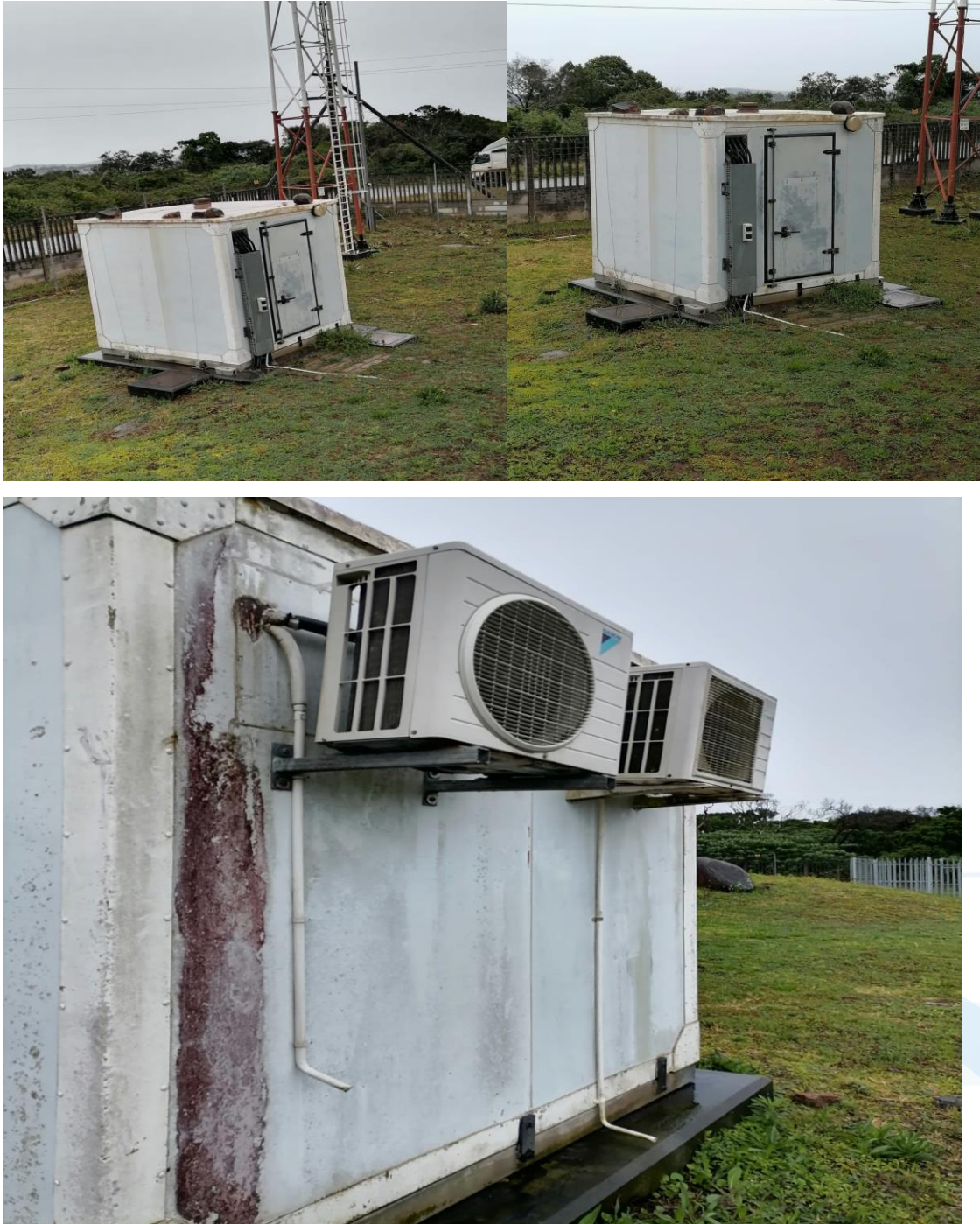
Figure 1: Examples of a transmitter container that requires refurbishment.
