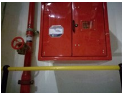
New hose reel + installation + new waterpipe and mounting bracket (see picture below)
