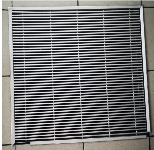
Figure 19. Example of air vent
