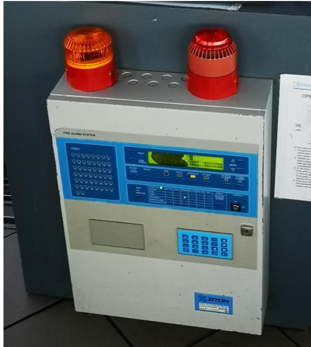
Figure 17. Fire alarm system panel
