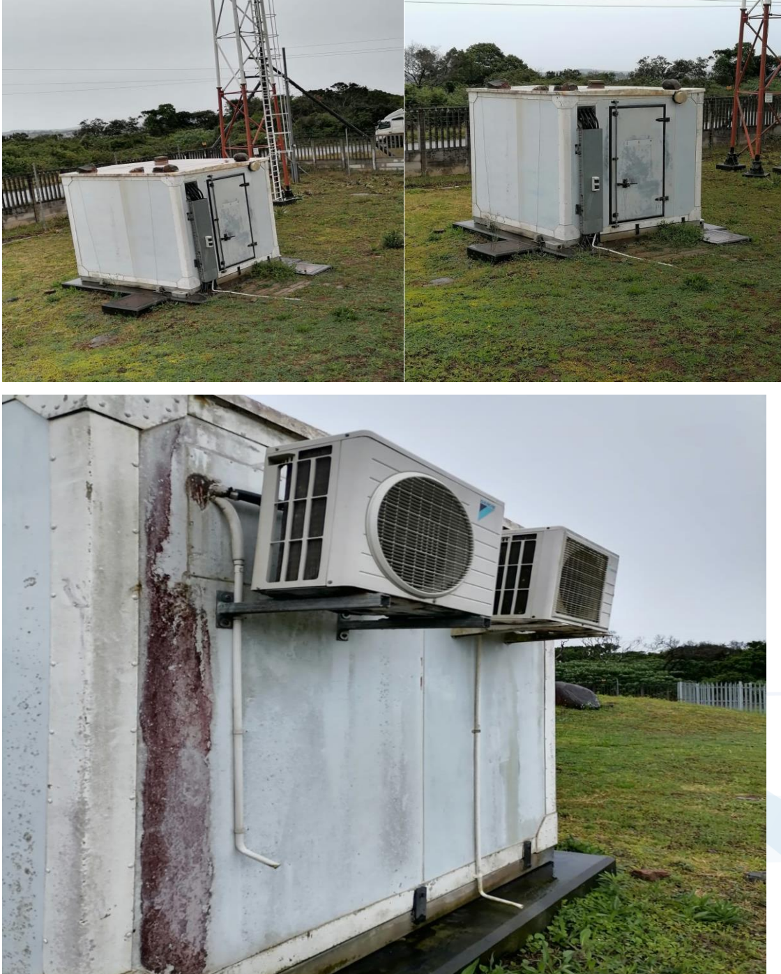
Figure 1: Example of a transmitter container that requires refurbishment.
